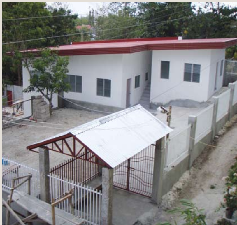
The construction works at Lola Daycare Center are now coming to an end.
